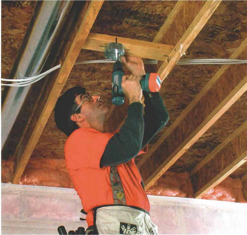
Wood and steel support ceiling fan. Mounted on the flat and secured to the joists with 3-in. screws, a recessed 2x4 block holds up the 2-in. deep metal box that supports the ceiling fan.
